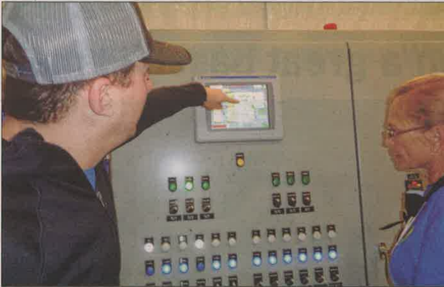
Adam Sommers, engineer with AquaWorks DBO Inc., and Ginger Bruvold, board member of the Florissant Water and Sanitation District, look over the computer that monitors the operations of the new wastewater treatment plant. Photo by Pat Hill
